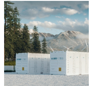
Battery Storage Power Station
