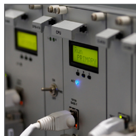
PLC/Motion Control Unit
