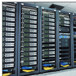
Data Center Switches
