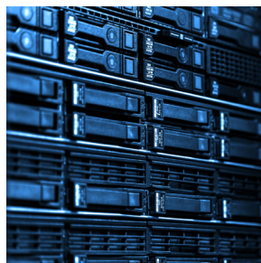
Data Center Servers
